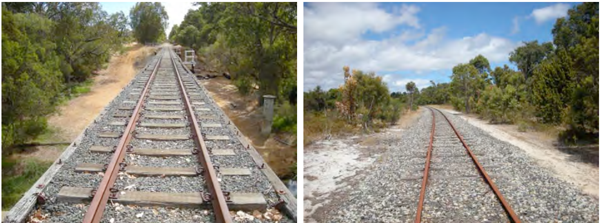
The railway bridge over the Capel River in Capel (left) would be a spectacular feature of the trail on the disused railway. The railway (right) has been unused for many years and there appears little chance that it will be reopened. 'Rail-trails' (trails built on disused railways) are a worldwide phenomenon.
