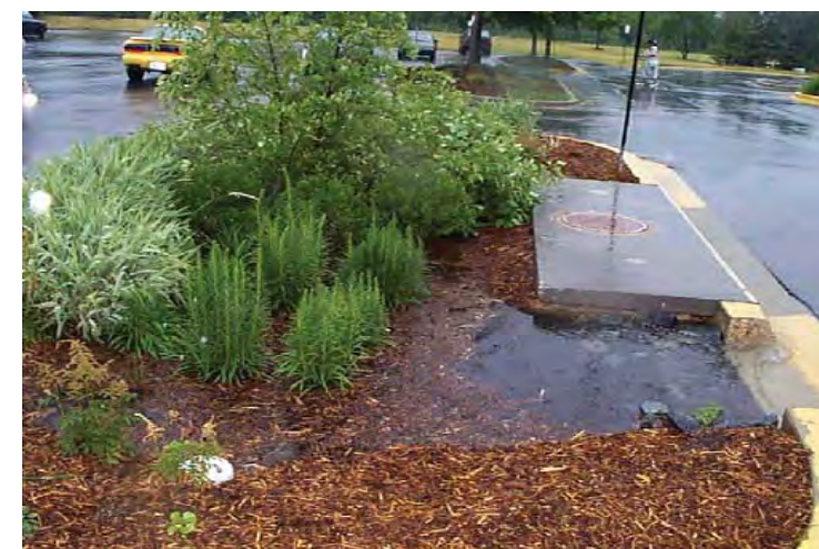
Road Bioretention unit at capacity
