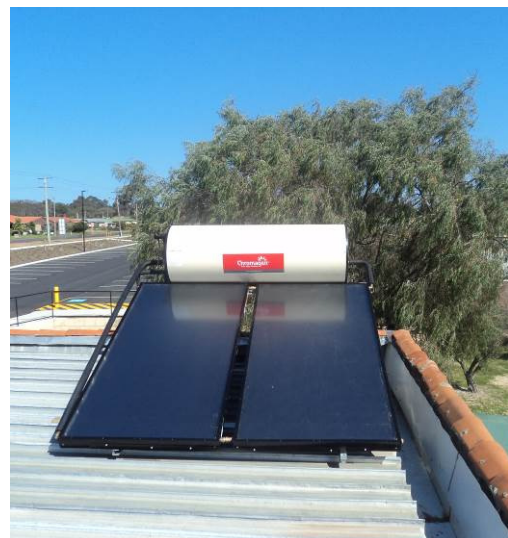
Gas-boosted solar hot water system at Capel Country Club
