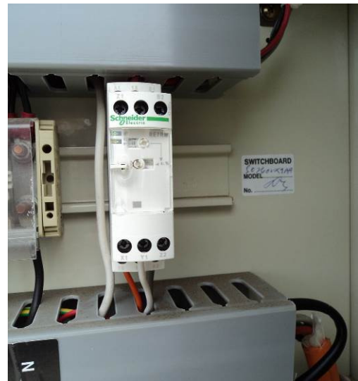
Timer control installed in air-conditioner at Dalyellup Community Centre
